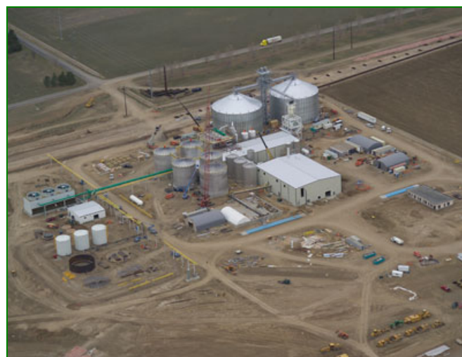
FRONT RANGE ENERGY PLANT
